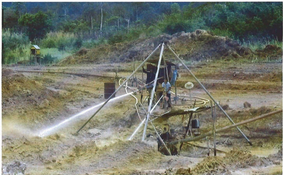
Figure 4. At Bo Rai, gem gravels are washed by high-pressure water cannons and transported up a pipe (seen to the right in photo) to a long sluice.
