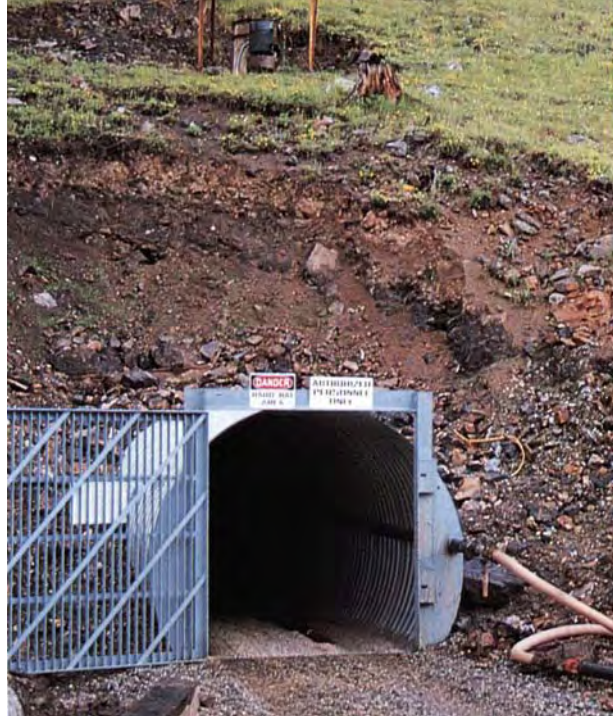
Figure 7. The Sweet Home mine is cold, wet, dark, at an extreme altitude, and absolutely inaccessible for all but a few months a year. This new portal leads to an extensive underground mine with slippery, vertical tunnels extending up sometimes 200 feet (61 m) high. Photo © Bryan Lees.
