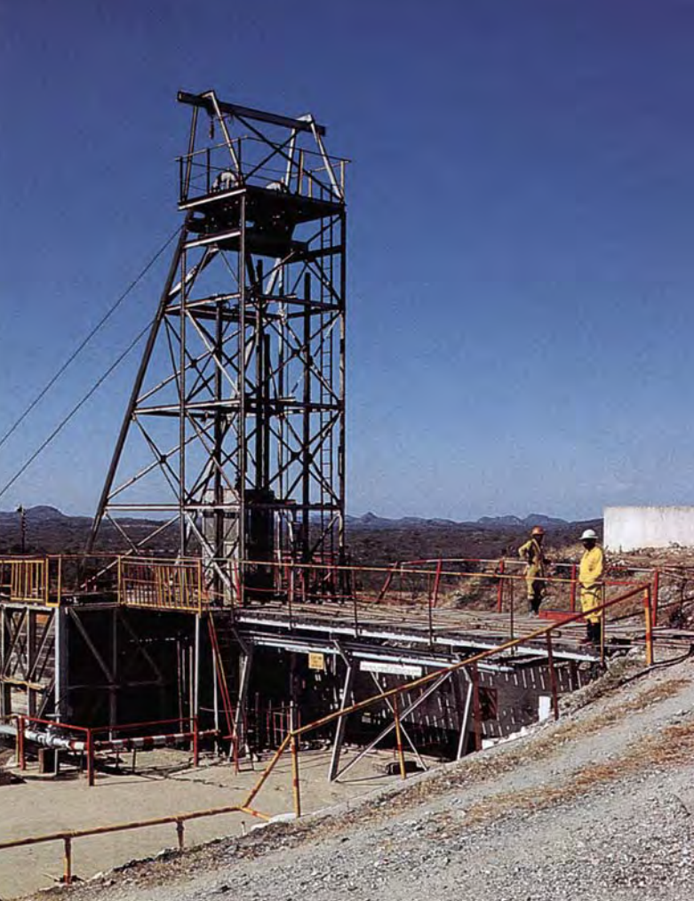
Figure 6. The main production shaft at the Zeus mine, the No. 3 shaft, serves as a haulage shaft down to 400 feet (122 m). Photo by E. J. Petsch.
