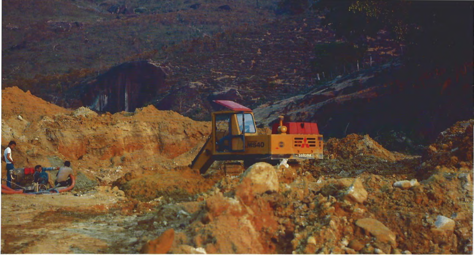
Figure 6. Here a backhoe is used to remove the red soil overburden and the first layer of black clay mixed with sand to get to the top cascalho layer (the yellowish material in front of the backhoe) at Barro Preto. Water is a threat to mechanized mining as well; note the pump on the left. The granite inselberg behind the operation may have been the original source of the chrysoberyl. Photo by Henry Kennedy.
