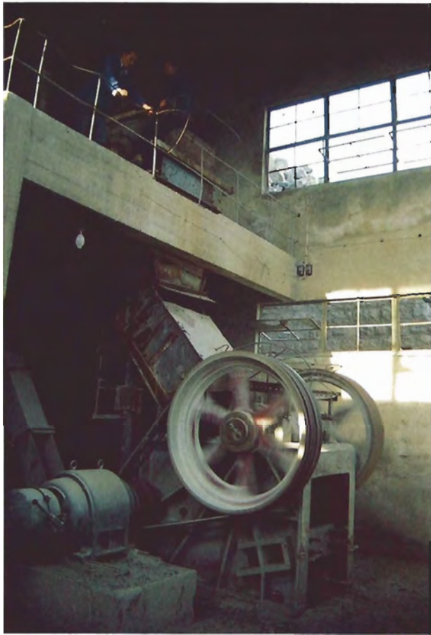
Figure 8. Ore from the Victory No. 1 mine first passes through a 15-cm "grizzly" and jaw crusher.
